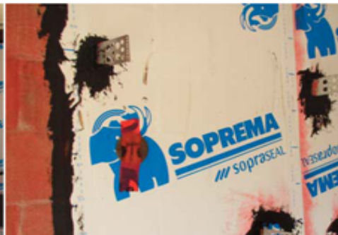
Masonry ties penetrate the wrap and must be sealed to maintain air tightness
