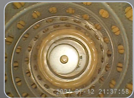
Oil Filter inspection using a E-Series Video Borescope
