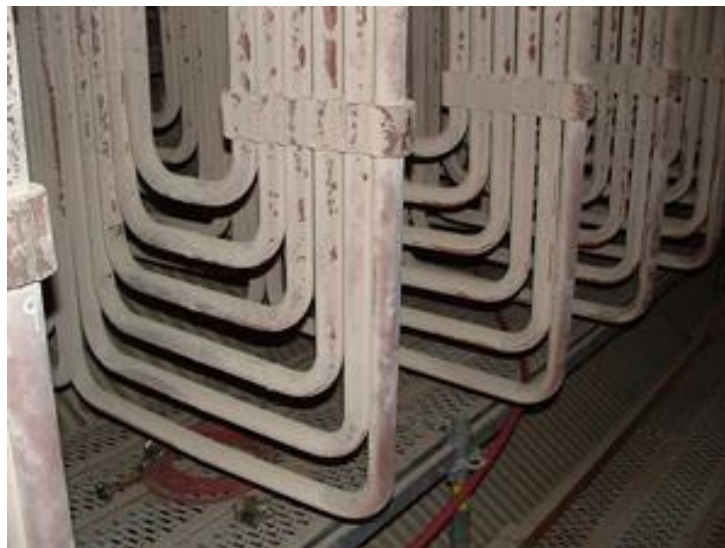
Pendant of Secondary Superheat Outlet Tubes
